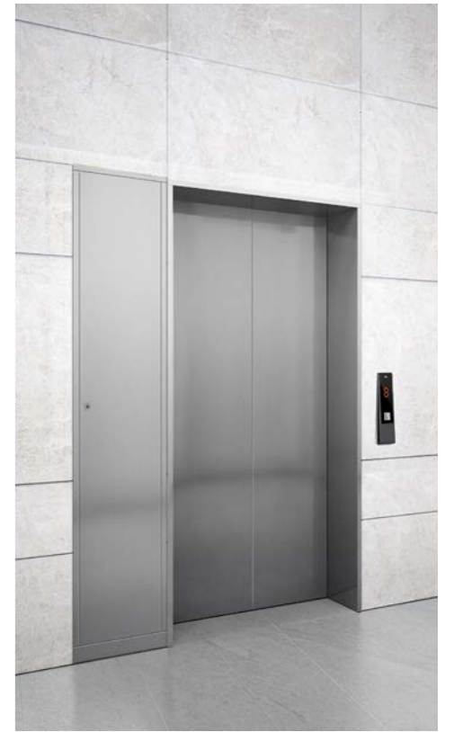
Entrance with control panel
