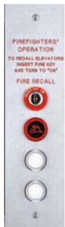
Intermediate hall station with fire services devices
