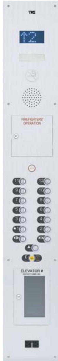
Car operating panel
