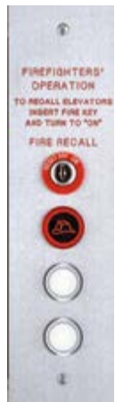
Intermediate hall station with fire services devices
